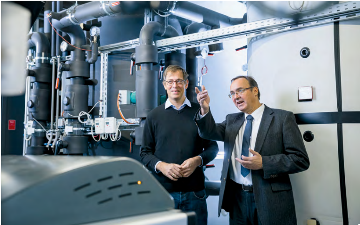
Prof. Rolf Bracke (right) and Gregor Bussmann discuss the project in the powerhouse of the geothermal center. © Sascha Kreklau/Fraunhofer
