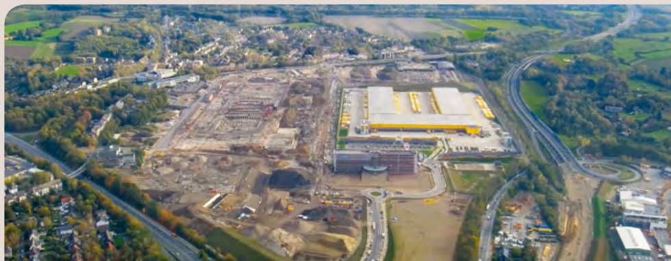
The former Opel site, covering 70 hectares: right, the new DHL parcel distribution center; left, construction of buildings for research institutes and tech companies, which are to be supplied with geothermal energy from mine water. © Lutz Leitmann
